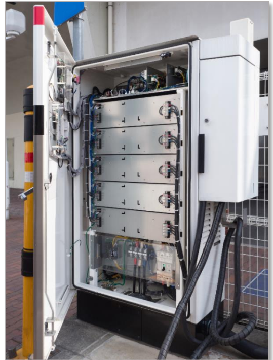
Cabinet for charging station
